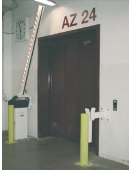
Barrier used to secure access to a freight elevator inside a plant
