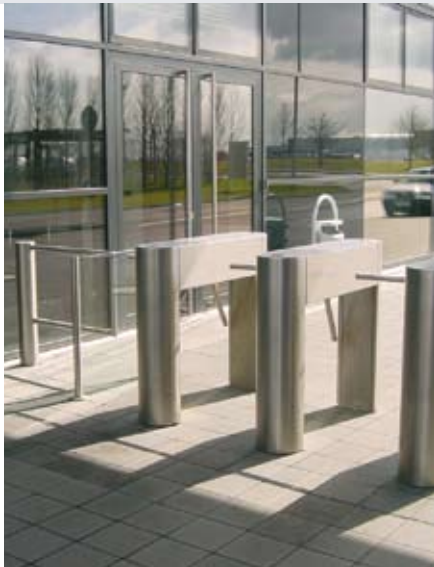
Access to company site, outdoor installation
